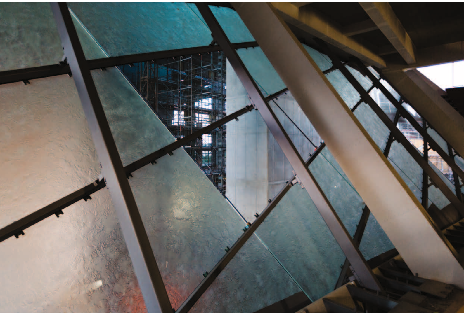
The eastern interior facade of the entrance building, which separates the press centre from the main lobby, consists of translucent glass panels mounted on a customised steel grid. The translucency of the glass panels is created by sandblasting the glass.
